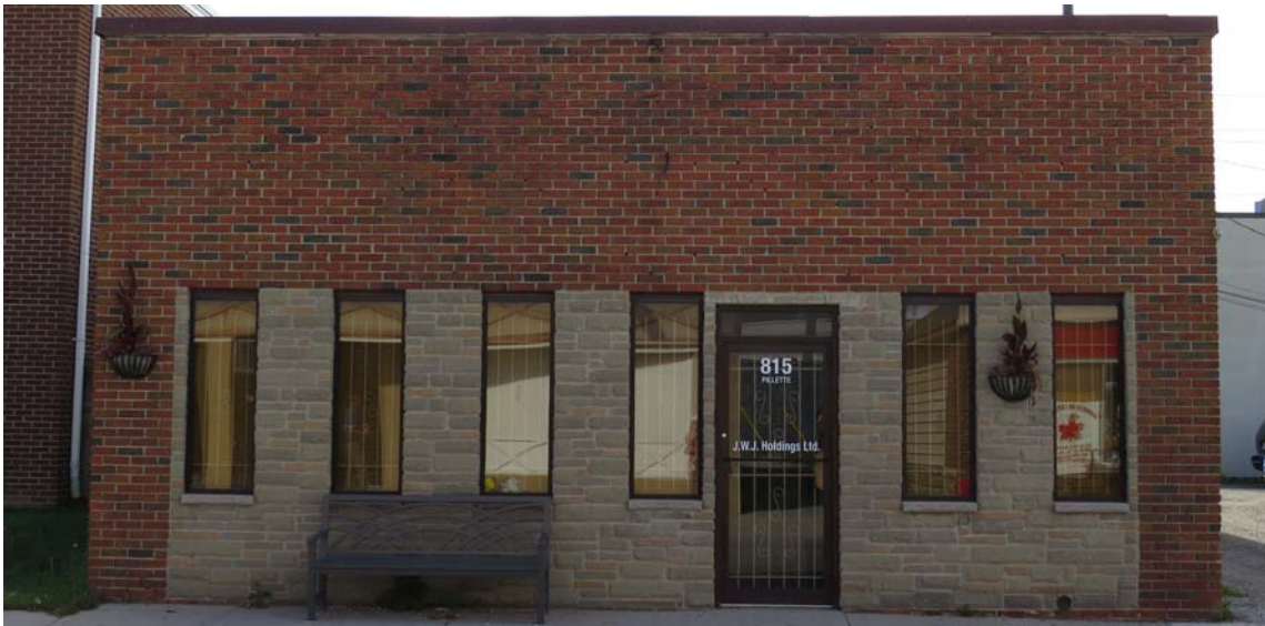
Figure 121. Windows have been removed and non-traditional materials fill in the original traditional Main Street storefront at 815 Pillette Road
