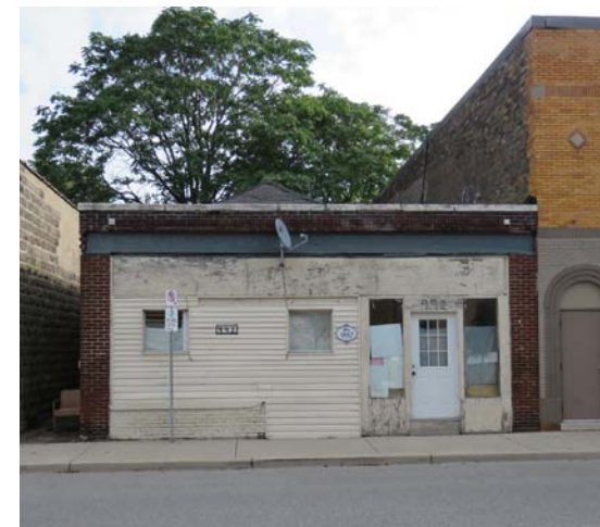
Figure 102. Example of a building in Ford City where storefront doors and windows have been boarded up
